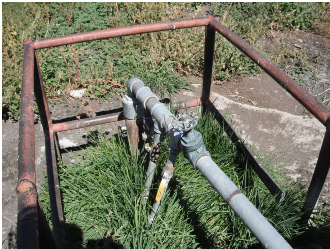
Plumbing associated with one of the artesian wells providing water to one of the water tanks in the southern animal corral.
