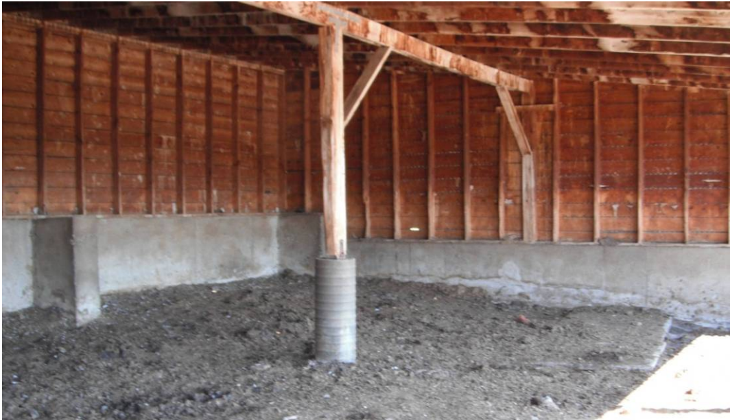
Looking at a structure used to provide shelter from the weather to animals near the southern animal corral.
