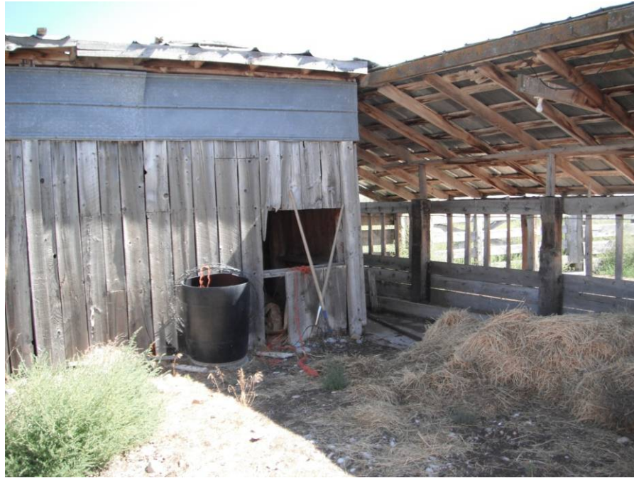
Looking at a storage shed and covering over the animal feeding area adjacent to the northern animal corral near the north central portion of the subject property.
