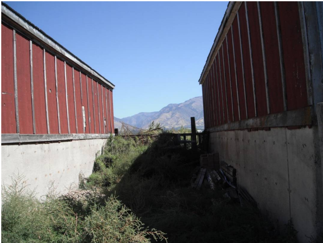
Looking east between two structures used to provide shelter from the weather to animals near the southern animal corral located in the south central portion of the subject property.
